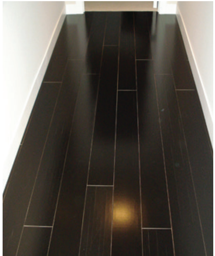
This engineered floor shrank after being exposed to low-humidity conditions, causing it to shrink on all sides and exposing the lighter color of the unstained board edges. Some face-checking is also evident.
