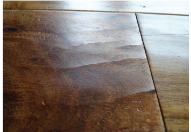
A wear layer held in place as it shrunk in low-humidity conditions led to face-checking on this wood flooring.
